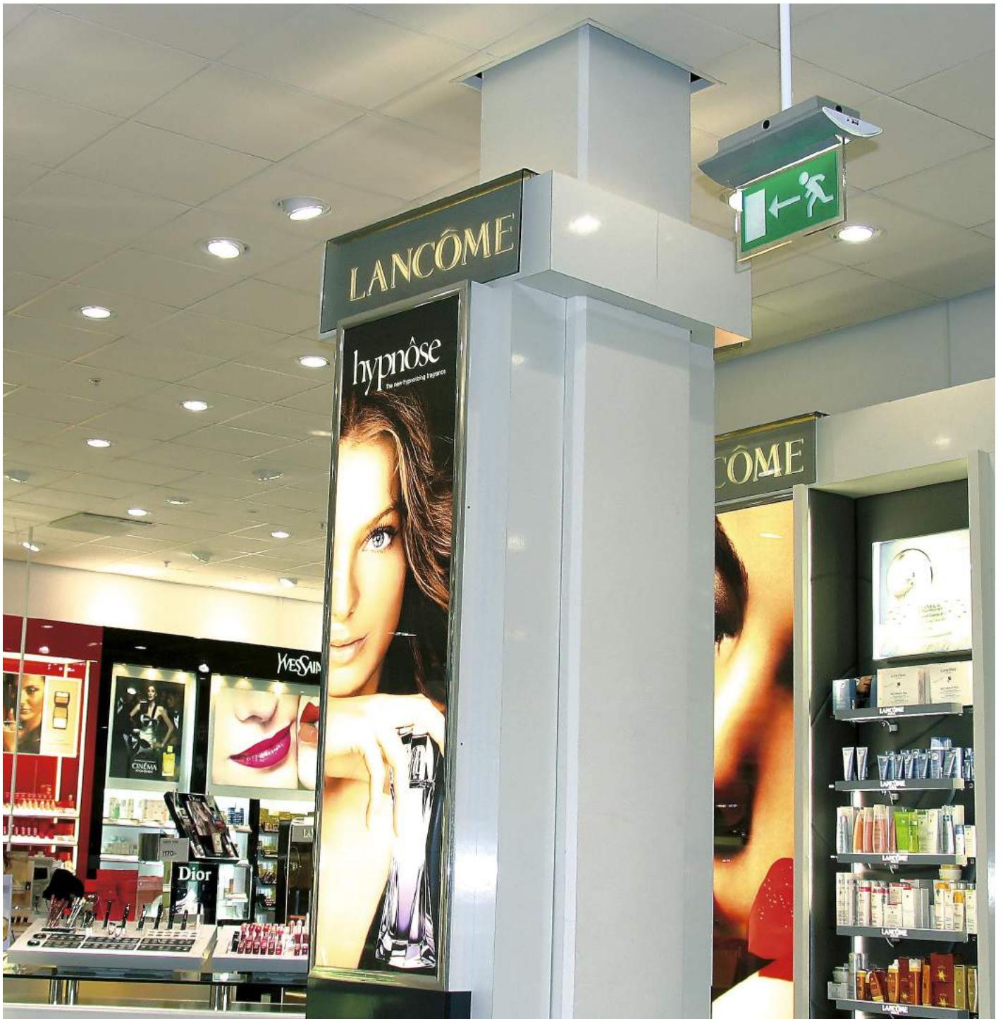
Shopping area emergency lighting application
