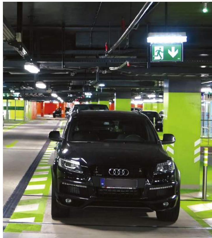
Parking Garage Area Emergency Lighting Application
