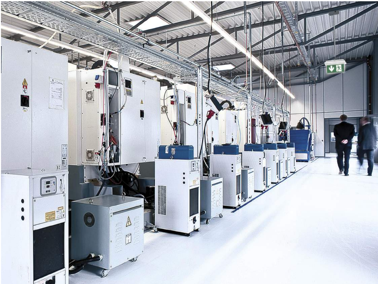
Industrial Area Emergency Lighting Application
